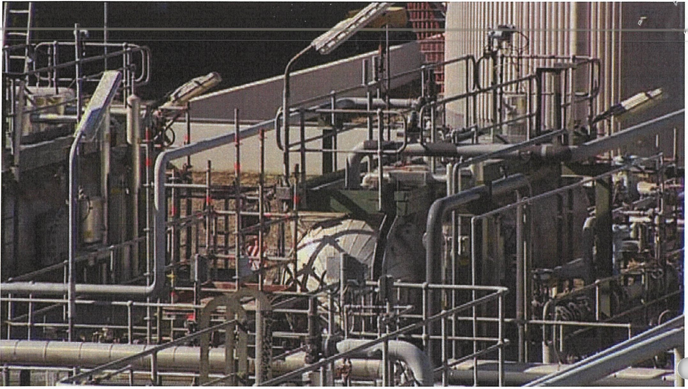
Todd Energy's Kapuni plant. (Source: 1News)
